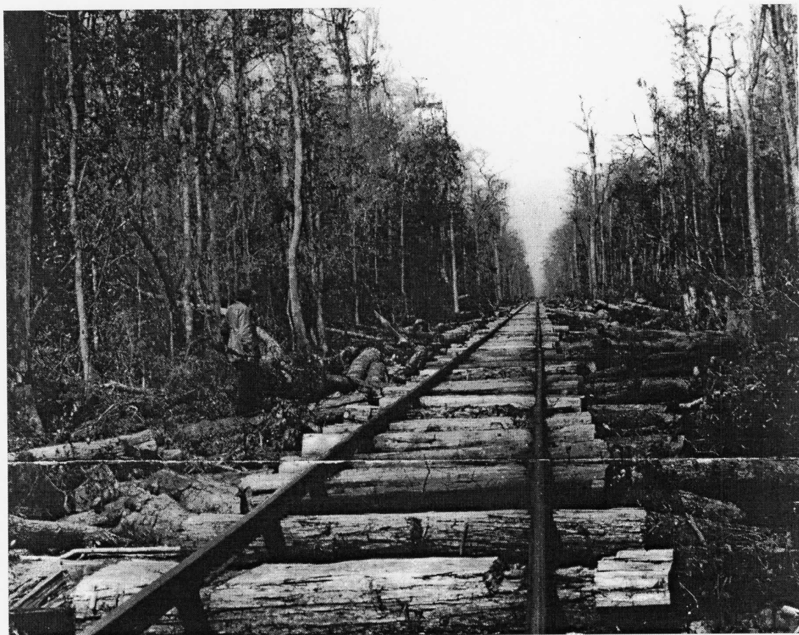
Main line in Okefenokee between the Swamp's edge and Cravens Hammock constructed with a pile driver - 10" caps (hewn 2 sides) fastened to piles with \frac{5}{8} iron drift bolts - 7 bents to 39-foot rail (Hopkins, 45 Years with the Okefenokee Swamp , 1947; RG-50-2-33, S.W. McCallie, March 1915, Georgia Department of Archives and History, Atlanta, Georgia).
