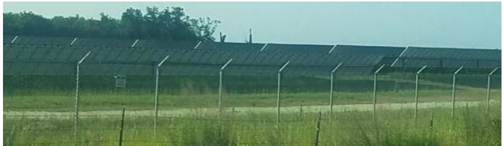
Photo: John S. Quarterman, 1 June 2019, of Duke Energy Hamilton Solar Farm, Hamilton County, Florida.
