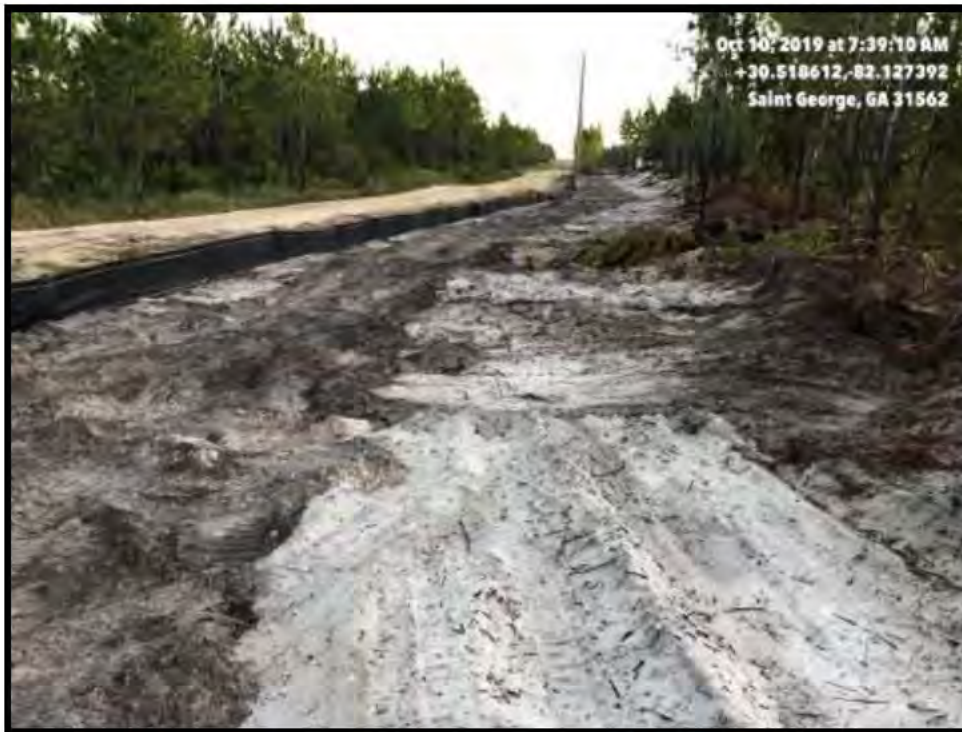
Photograph 4: View to the north of T-Model Road, silt fence, and cleared vegetation.
