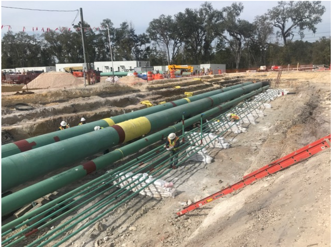
Dunnellon Compressor Station: (facing Northeast)
