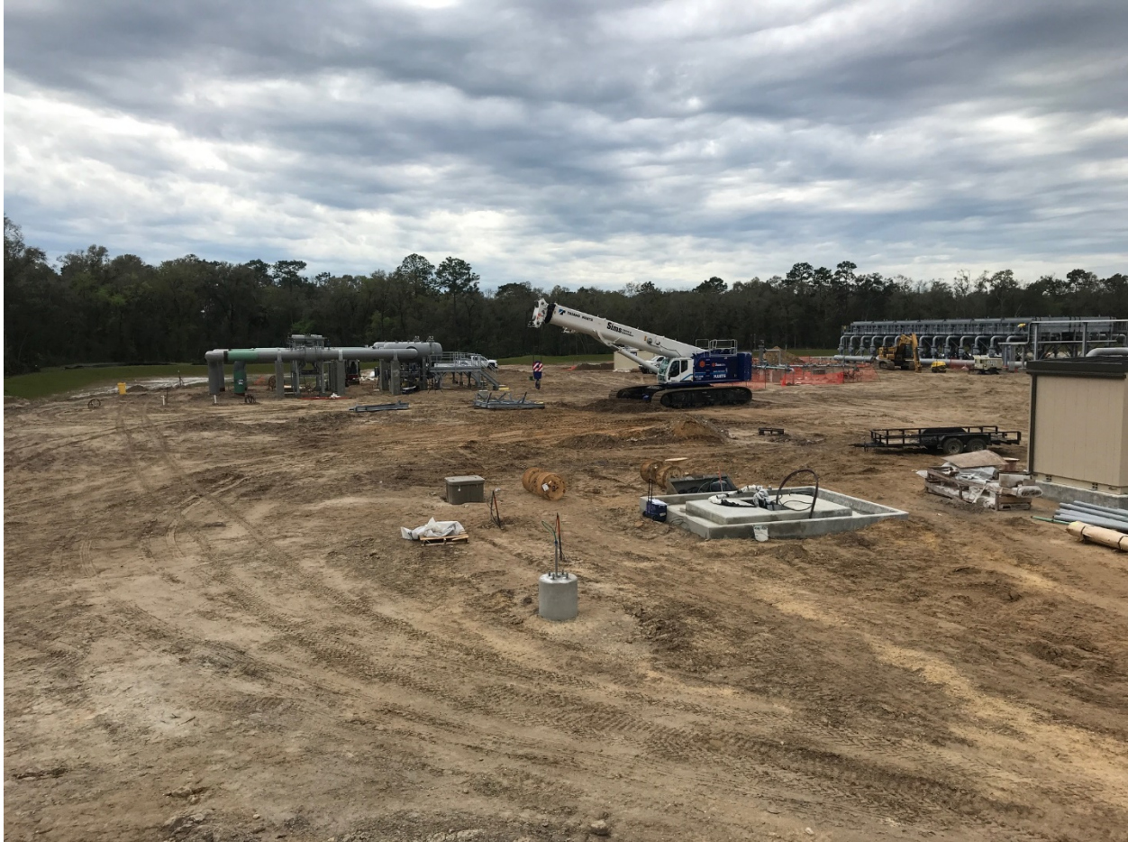
Dunnellon Compressor Station: (facing South)
