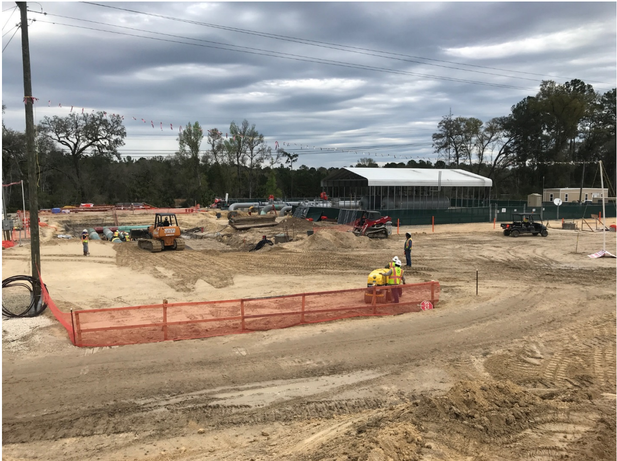
Dunnellon Compressor Station: (facing North)
