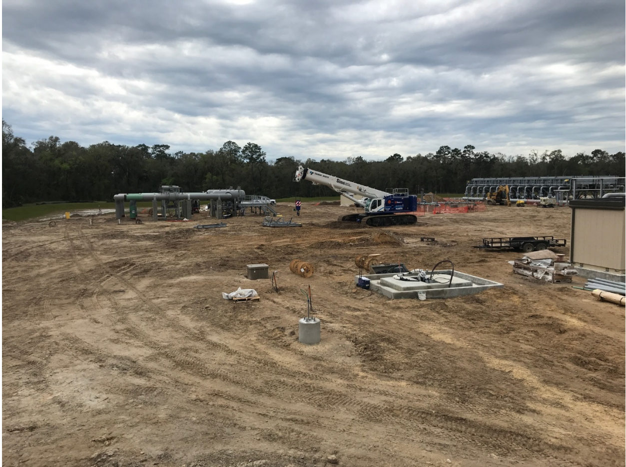
Dunnellon Compressor Station: (facing South)
