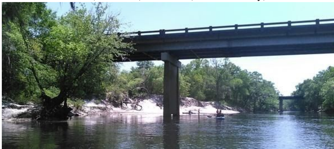
Photo: John S. Quarterman for WWALS, Howell Road Bridge and Mayday Landing, 2016-05-07
