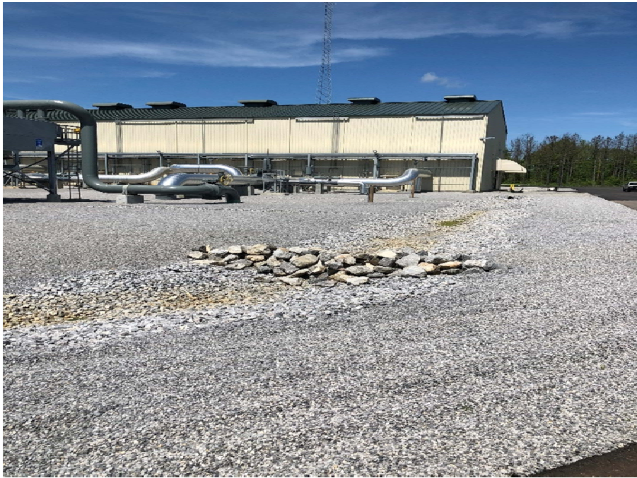
Photo 17: Station 95. View of permanently stabilized area around the new addition to the east side of the facility on 3/25/2020. Facing north.
