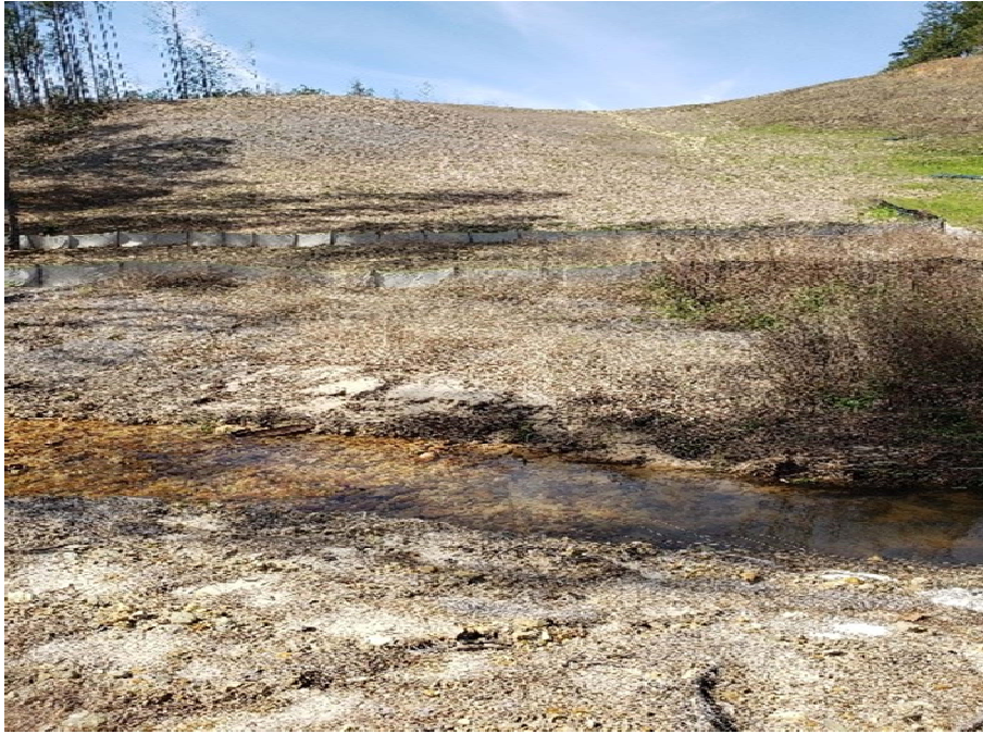
Photo 1: Rock Springs Loop. Overview of restored right-of-way around the SCW9C001 stream crossing on 3/7/2020. Facing west.
