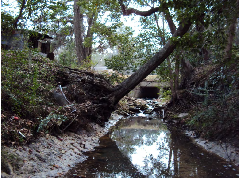
Figure 3.3.11. Knick Point about 400 feet Downstream of W. Magnolia Street
