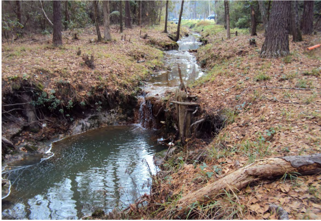
Figure 3.3.4. Knick Point 250 feet Downstream of River Street
