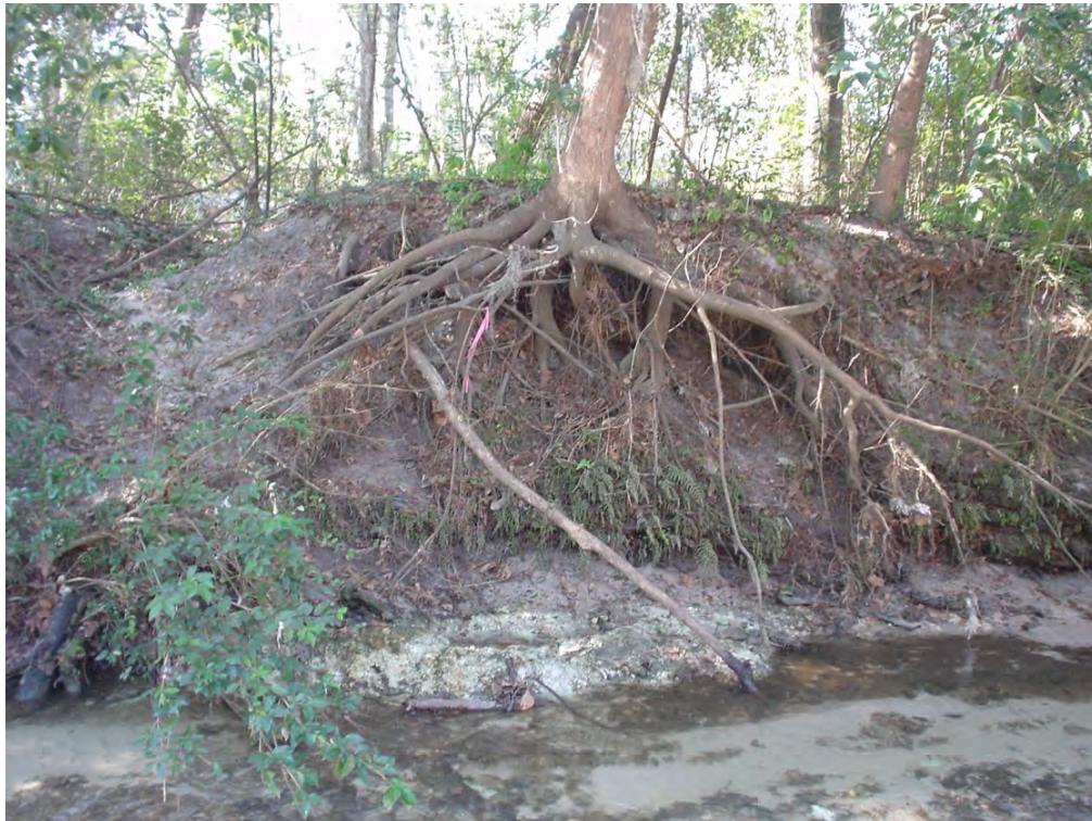
Figure 3.3.20. Incision has let to Vegetation Damage
