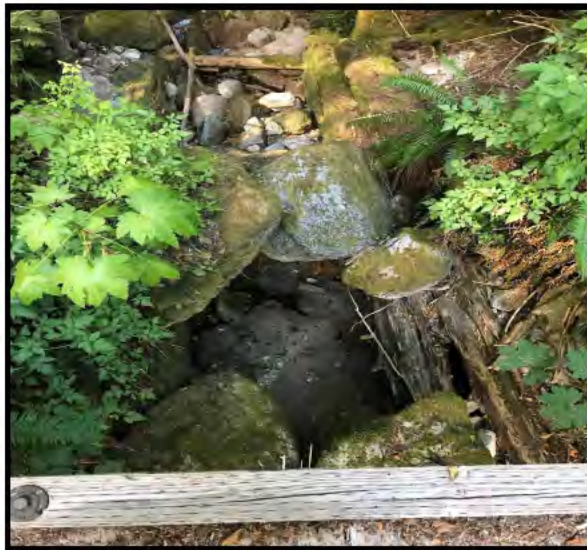
A trickle of water emerges beneath a footbridge Footbridge, tributary to Middle Fork Snoqualmie River. Photos: 2017, Chris Wilke
