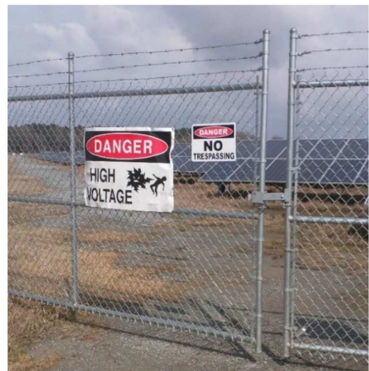
Figure 1. Perimeter Fence with Warning Signs
