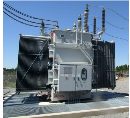
Figure 6. GSU Transformer with Secondary Containment to Capture any Leaked Oil
