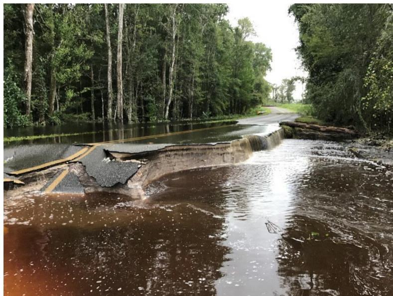
Roadway damage cause by erosion due to flooding during Hurricane Irma, 2017 – Bradford County File Photo
